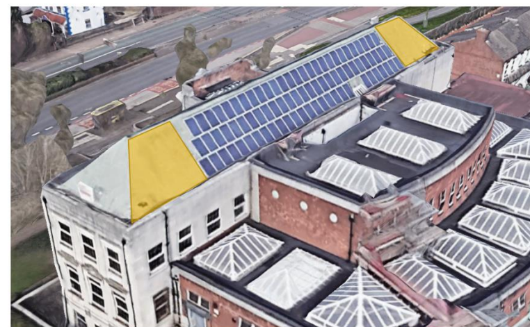
Existing PV system and rooftop areas suitable for solar PV highlighted, subject to structural survey.
